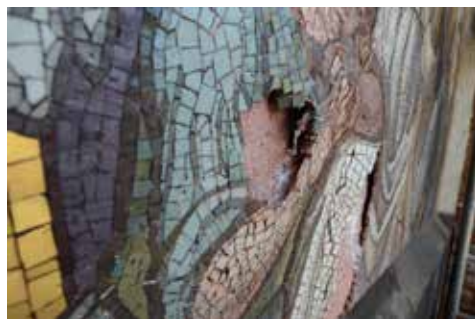
Fig. 1. Deformations and losses of the mosaic before application of the emergency facing, 2018 (photo by B. M. Kürtösi)
